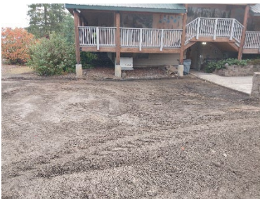
Preparing the area around the Weippe Public Library for asphalt application. Old railing still in place.
