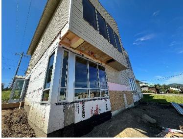
The exterior of the St. Maries Public Library building during its 2024 expansion.
